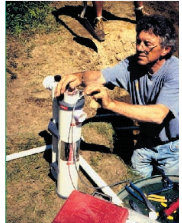
An ultraviolet light disinfection unit further reduces bacteria following the treatment unit. It typically fits into the pump chamber where treated effluent is pressure dosed to the drainfield for final dispersal.
