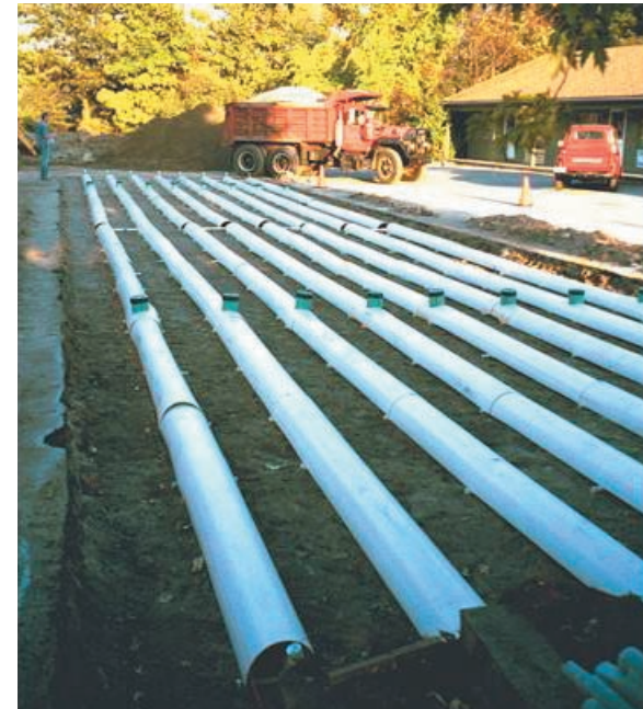
A shallow, narrow drainfield showing the outer PVC pipes that cover the pressure laterals. This drainfield serves a 2700 gallon-per-day restaurant and retail / office complex. These lines, located in a parking lot island, are ready to be covered with native backfill, and will be 12" below finish grade.
