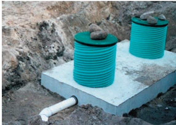
The picture above shows a concrete tank with access risers above inspection ports. When backfilled, riser lids will be at ground surface.
