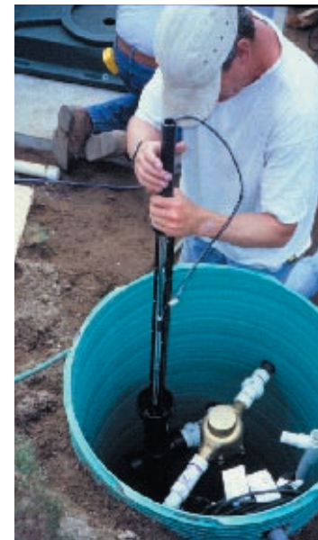
A pump chamber. This may also house recirculating valves, timers and other controls. The finished unit will have a green lid at the ground surface.
