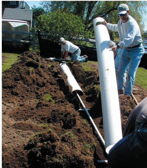
Installation of a shallow, narrow drainfield. Pressurized laterals (1" diameter PVC pipes) are shielded with 12" PVC pipe cut lengthwise, with at-grade inspection ports located at regular intervals. Shallow narrow drainfields take advantage of biochemically-active upper soil layers for microbial nutrient removal and plant uptake.
