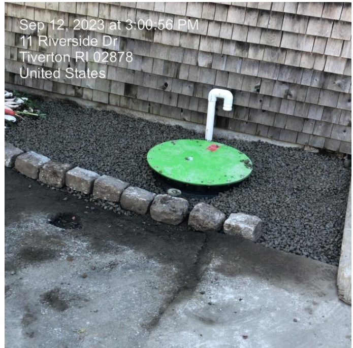
Figure 1 Typical grinder pump installation at surface.
